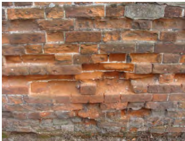
Picture 1.18 Garden wall to The Grange, Church Street, in urgent need of repair
